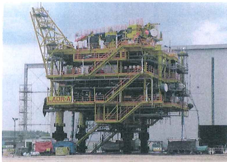
TH Heavy carries out fabrication work at its 58-acre yard in Pulau Indah, off Port Klang
